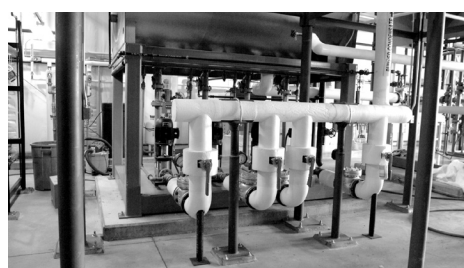
The pumps used in the condensate and boiler water treatment equipment in Building 359.
