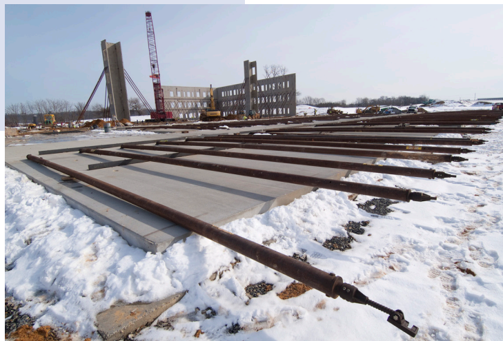
Braces are attached to the panels while they are still on the ground.
