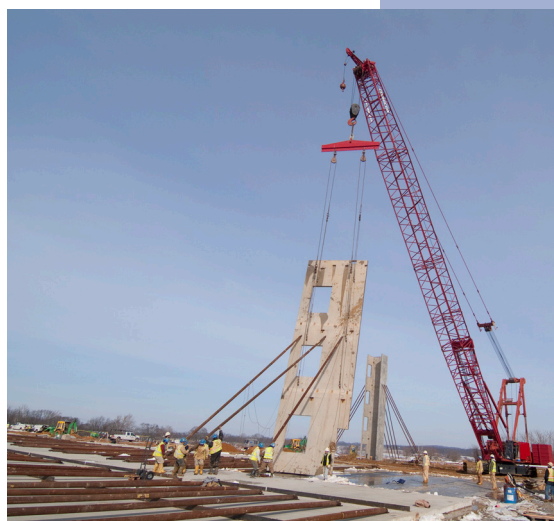
Using the braces, workers guide the panel while a mobile crane lifts it away from the ground. Each panel weighs approximately 35 tons, according to Todd Hiltner, Construction Manager, Facilities Maintenance and Engineering.
