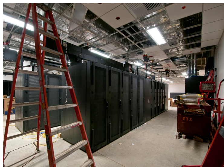
Interior fit-out in progress. Top: Laboratory on third floor; Bottom: Data center nearing completion, with server racks in place.
